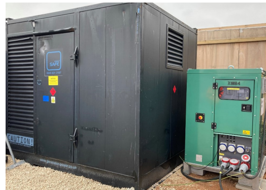
60KVA generator (left), 45 kW battery pack (right)
